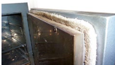
Figure 26 Asbestos rope seal on drying oven
