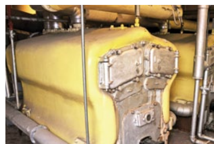
Figure 13 Amosite lagged boiler with hard plastic coating
