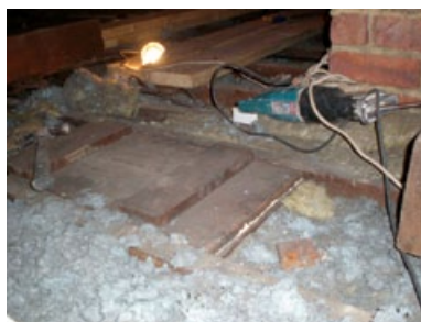
Figure 6 Loose asbestos used as loft insulation
