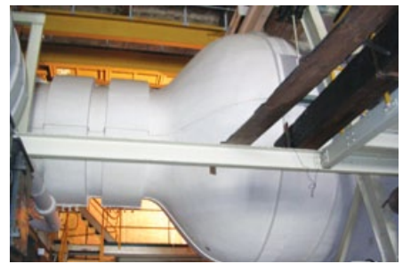
Figure 51 Vessel clad in amosite insulation
