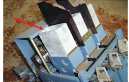
Figure 49 Electrical switchgear with asbestos flash protection
