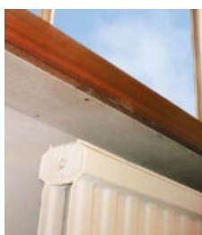
Figure 20 AIB panel between radiator and window
