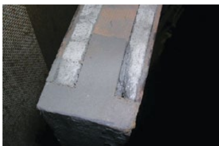
Figure 14 Asbestos panels inside fire door
