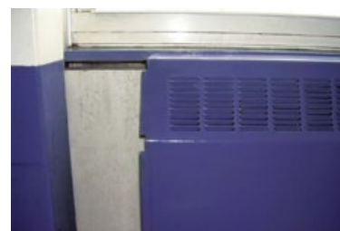
Figure 19 AIB behind school radiator unit
