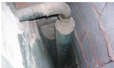
Figure 9 Lagged pipe in wall cavity
