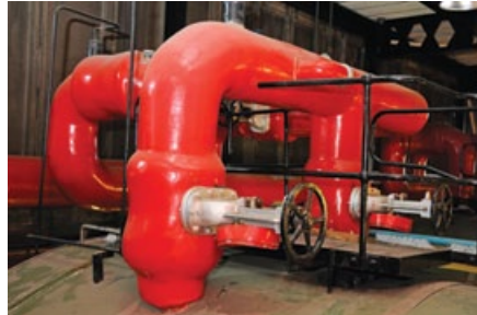
Figure 48 Asbestos-insulated supply pipes
