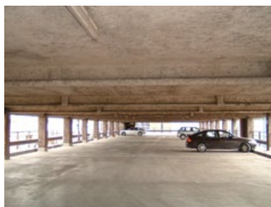
Figure 7 Sprayed limpet on car park roof
